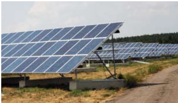
Electrical design in the solar park: 43,320 solar modules laid out in 1,805 strings. 14 central inverter stations. Each has a transformer station. The length of the cables from the string-monitors to the inverters is 175 km, from the modules to the string-monitors 375 km.
