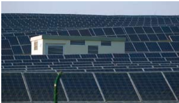
Electrical design in the solar park: 27,350 solar modules laid out in 1,302 strings. 5 central inverter stations of SMA (total AC capacity 5.0 MW). Each has a transformer station. The length of the 20 kV-cable to the grid-point is 1,5 km.
