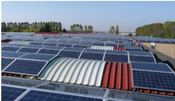
The specific shape and style of the roofs were also considered in the electrical design. In order to secure the light incidence into the halls, the light-transmissive parts of the roof were left open.
